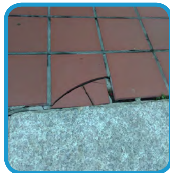
Over time, standing water and freeze-thaw cycles had cracked landing pavers and deteriorated mortar joints.
