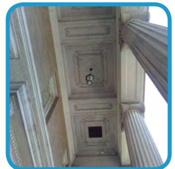
The three-story high plaster soffit had begun to crack and shed its paint finish.
