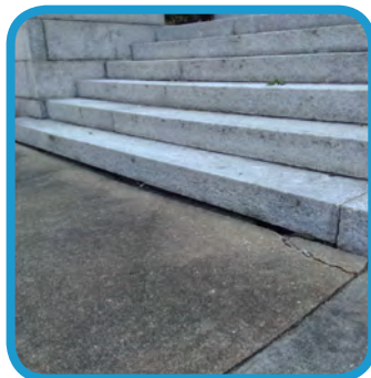
The gap between the concrete walk and the stone stair riser had become a tripping hazard.
