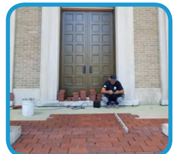
Terra cotta pavers were removed and replaced on both landings, including a new, upgraded setting bed and new mortar joints throughout.
